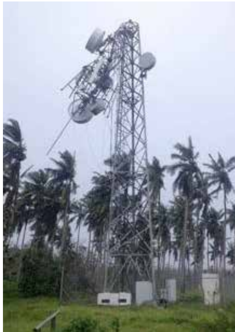
A mobile phone and communications tower located in Vanuatu, damaged by one of this years cyclones. Image by: dailypost.vu
